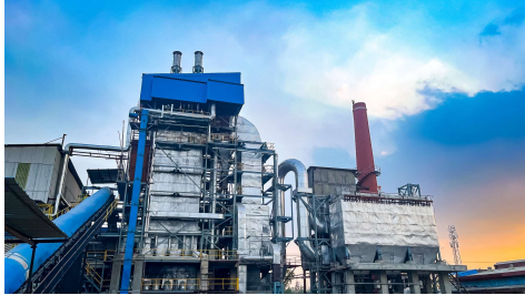
A typical image of multi-waste boiler
